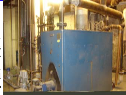
Logan Gardens boiler before repairs.
